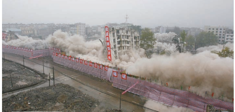
Above: Entire city blocks are razed to make way for the Three Gorges Dam in China
